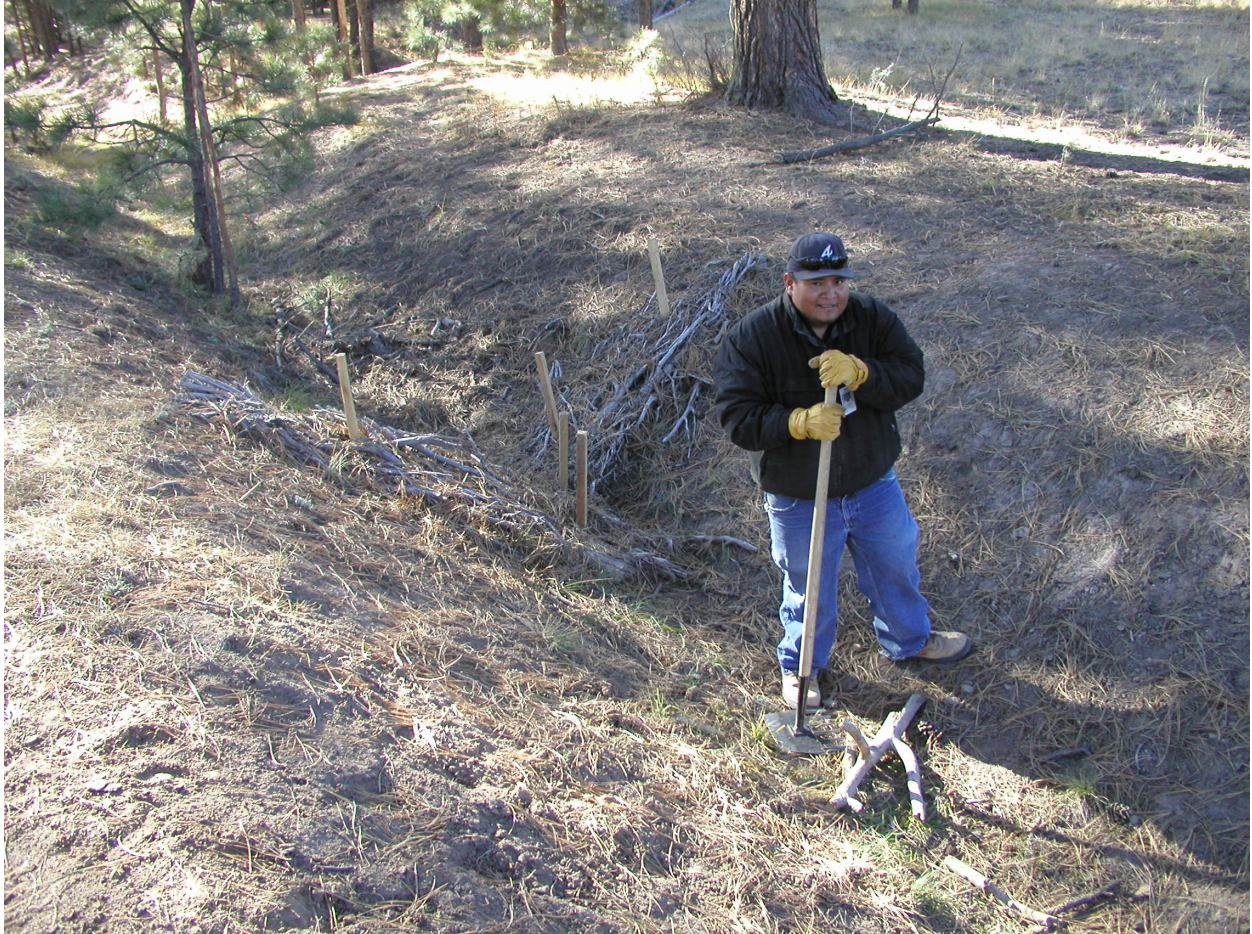
Figure 5 Juniper bale check dam in channel draining to 90s Line Pond repaired in November 2011
