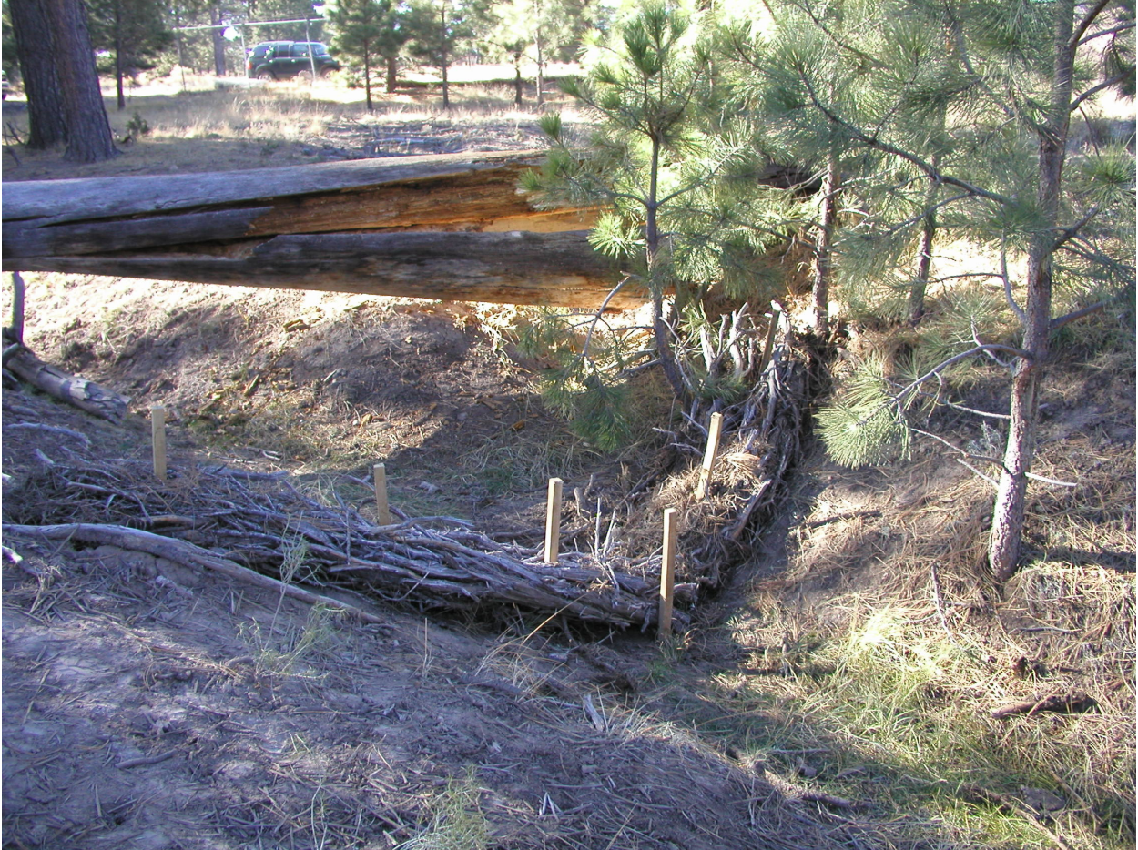
Figure 3 Juniper bale check dam in channel draining to 90s Line Pond repaired in November 2011
