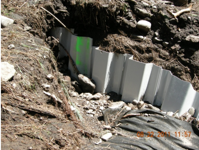
Damage occurred at the Permeable Reactive Barrier (PRB) in Upper Water Canyon from storm events on August 3 and August 21
