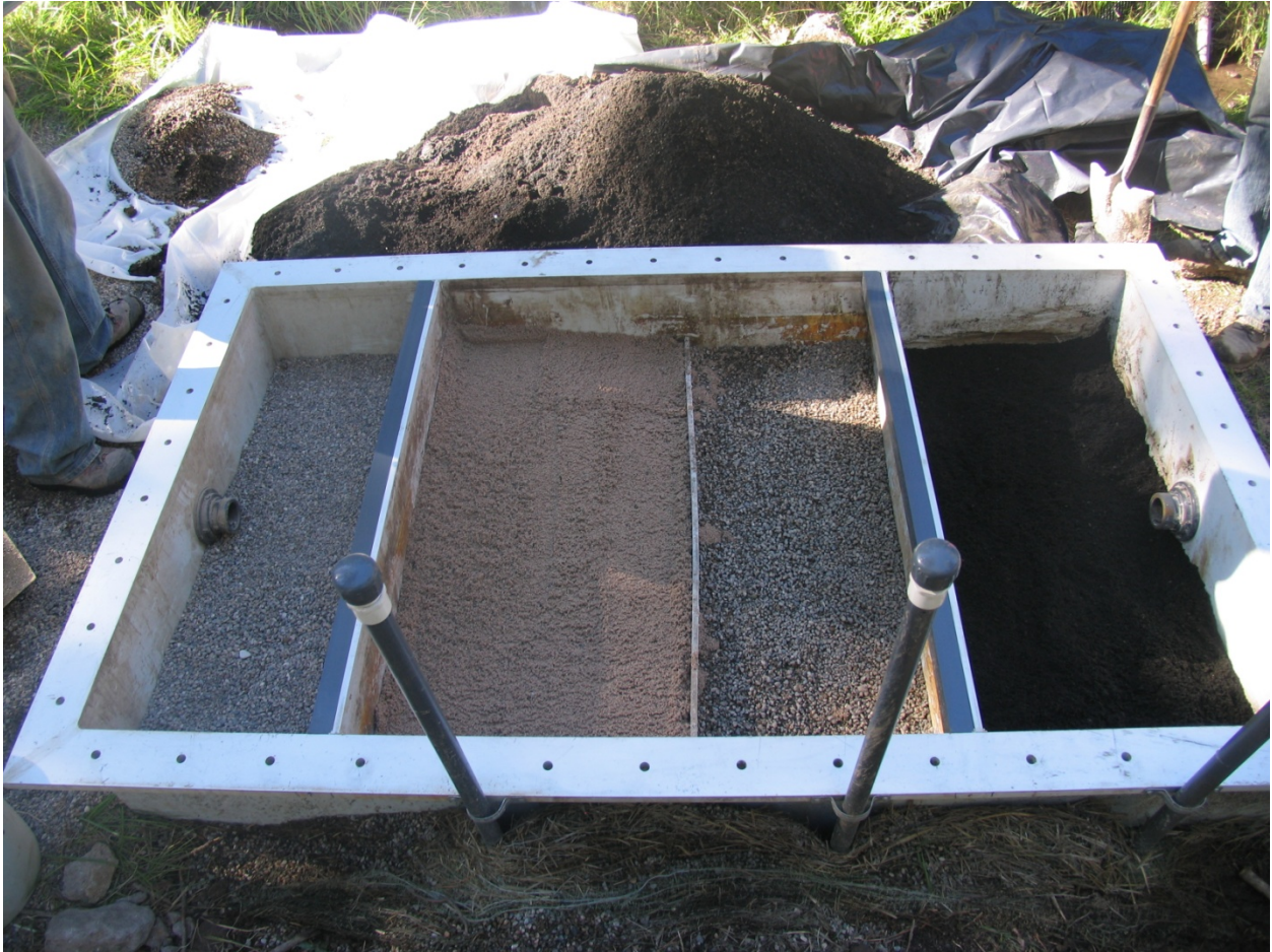
September 10, 2010: Second configuration: gravel, zeolite, gravel, ZVI. Reinforced baffles installed to prevent bypass.
