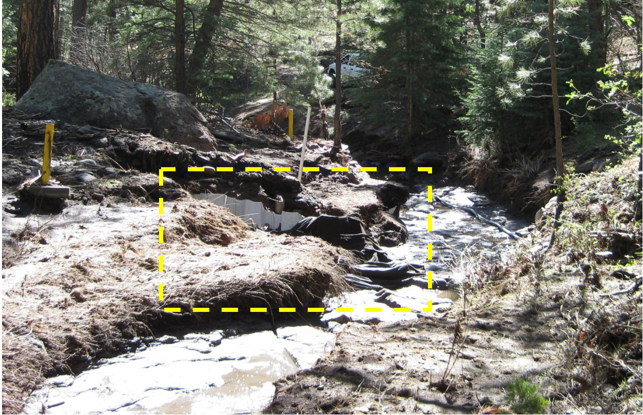
August 23, 2011: Post-8/21/11 flood. Cañon de Valle channel scoured to bedrock upgradient of PRB cutoff wall. Photograph shows remnants of PRB cutoff wall (geotextile, exposed piping in channel).
