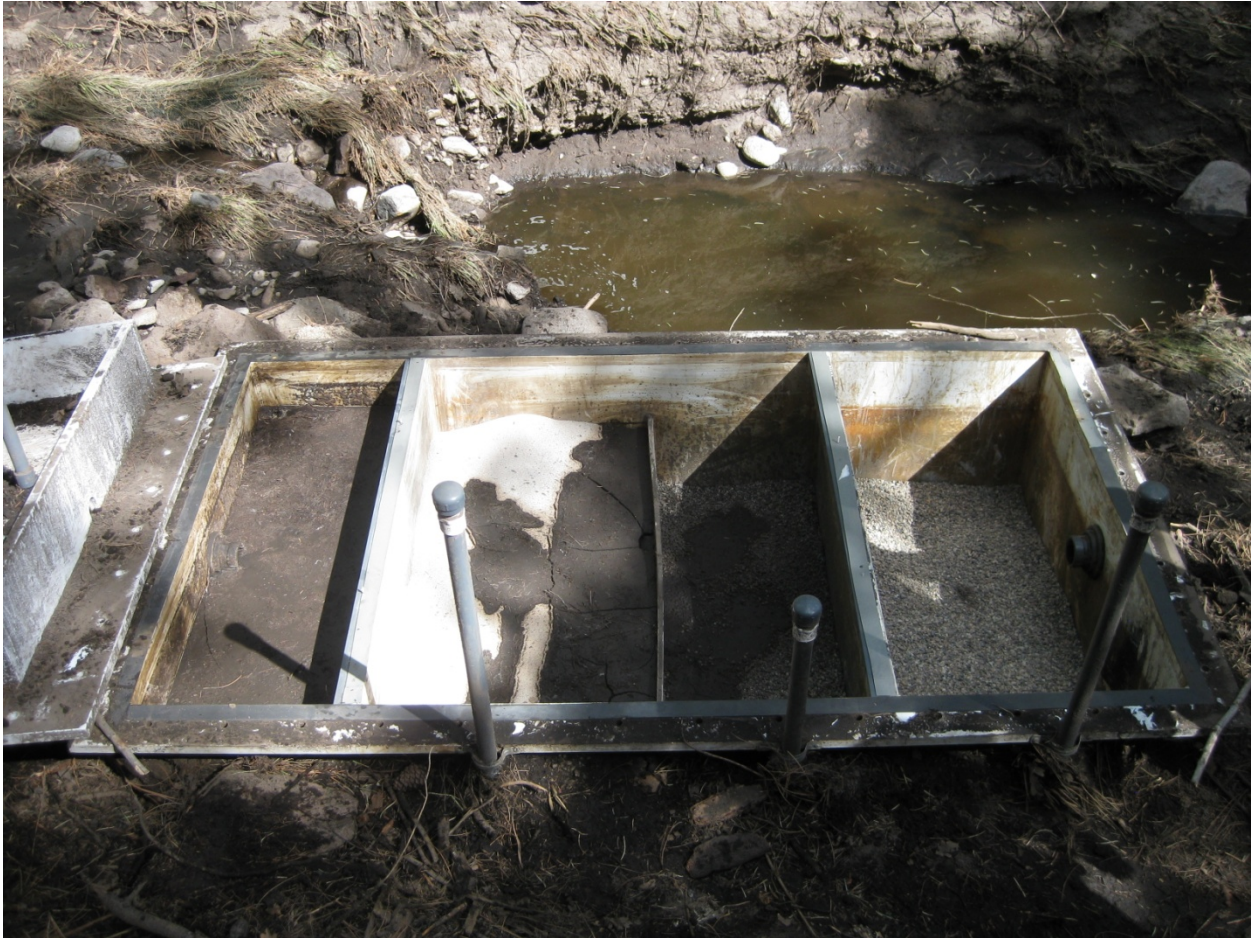
August 9, 2011: Post-8/3/11 flood damage. Input of stormwater and sediment to the vessel.
