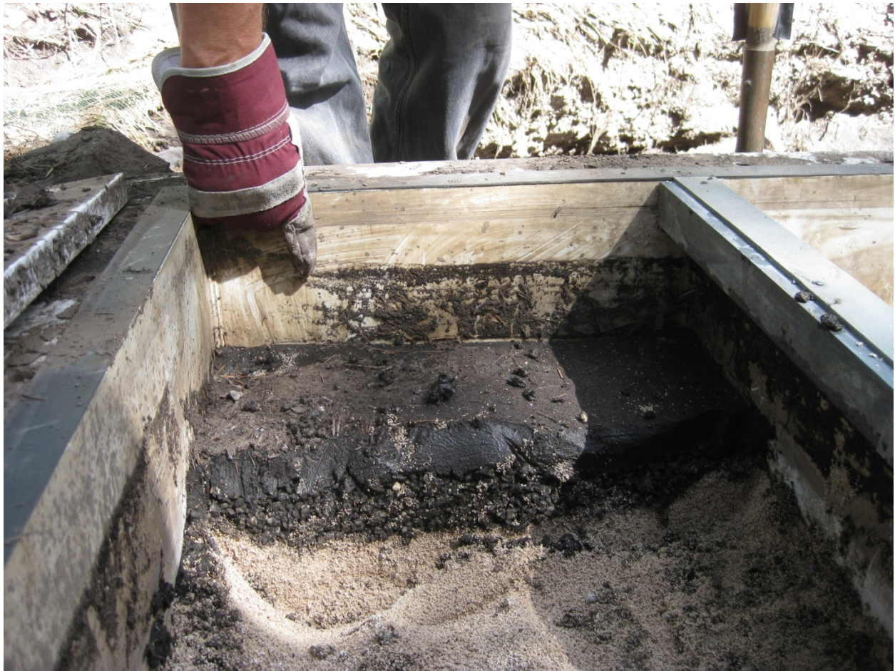
August 9, 2011: Post-8/3/11 flood. Cell 1, approximately 2 in. of ash and silt deposited on zeolite. Also note the high water mark of organic debris.
