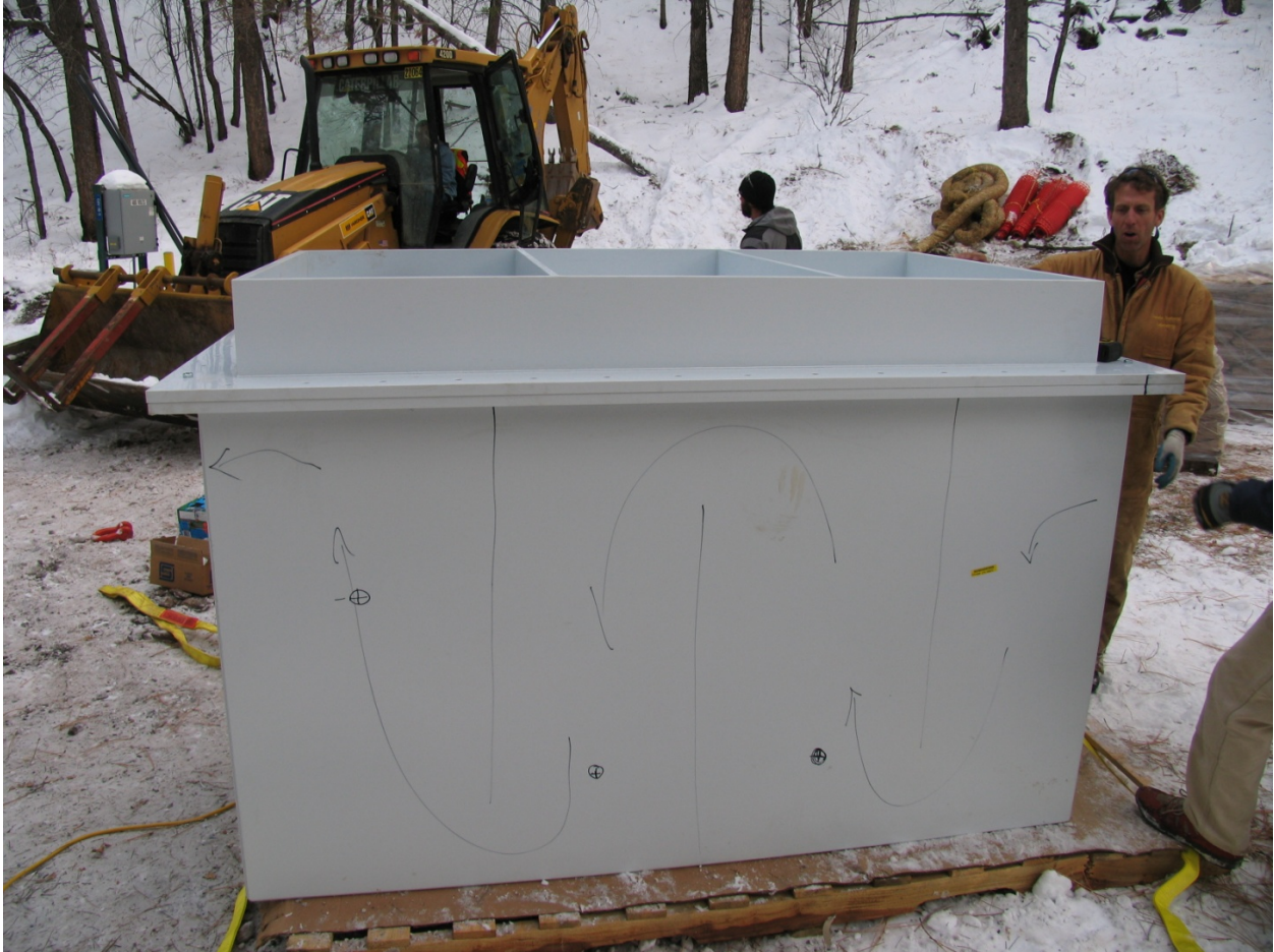
December 2009: Permeable reactive barrier (PRB) vessel before installation showing baffles and sample port locations.
