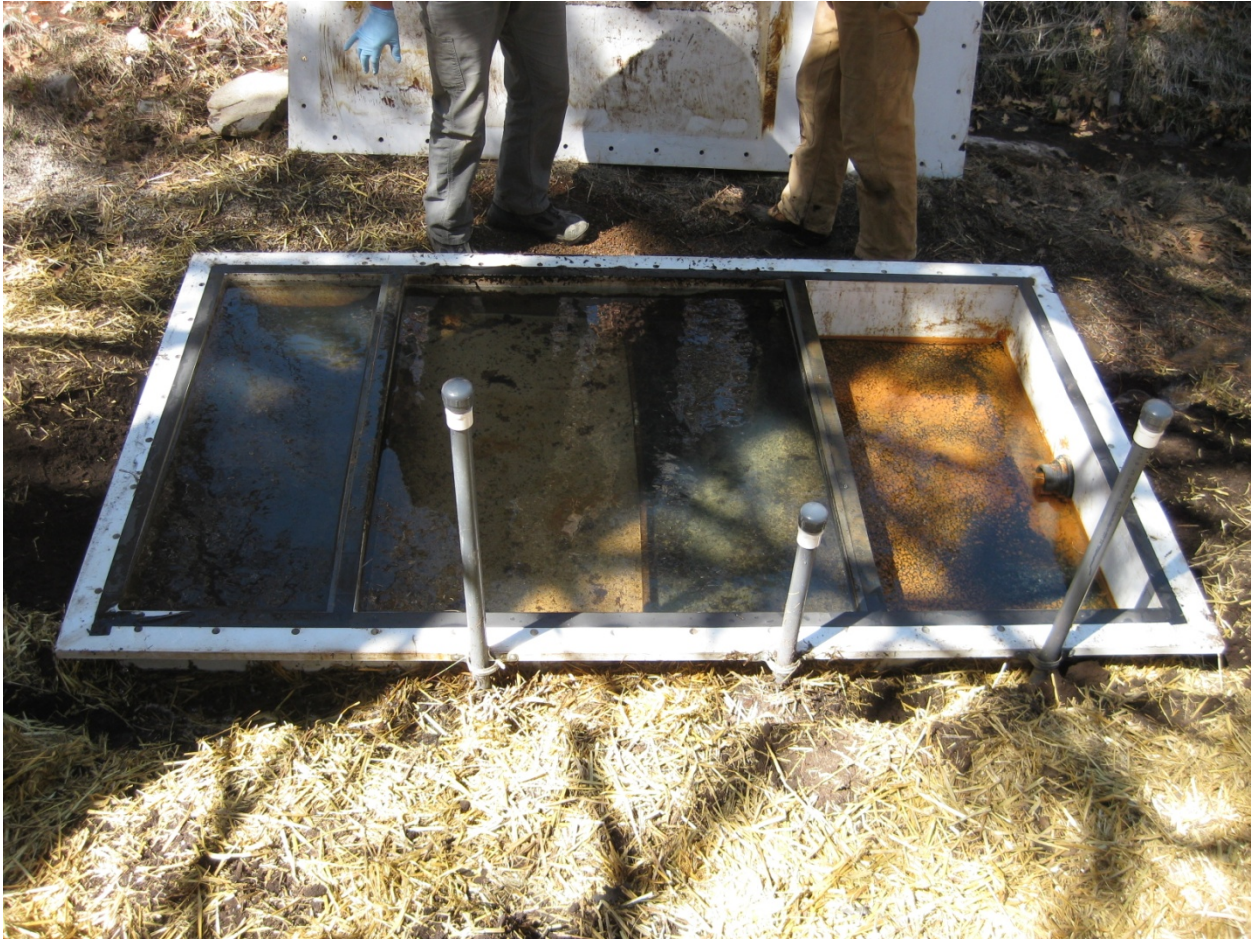
March 23, 2011: Configuration 2 assessment: gravel, zeolite, gravel, ZVI. No flow through ZVI chamber. Flow to the vessel backed up and eventually forced through the gasket at top of baffle.
