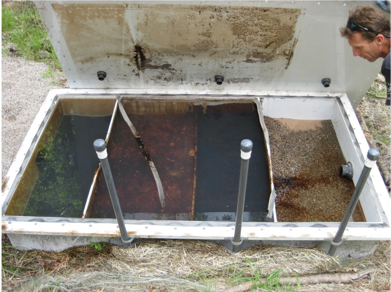
August 3, 2010: Reconfiguration: gravel, ZVI, gravel, zeolite. Bypass over baffles because of precipitation in ZVI chamber.
