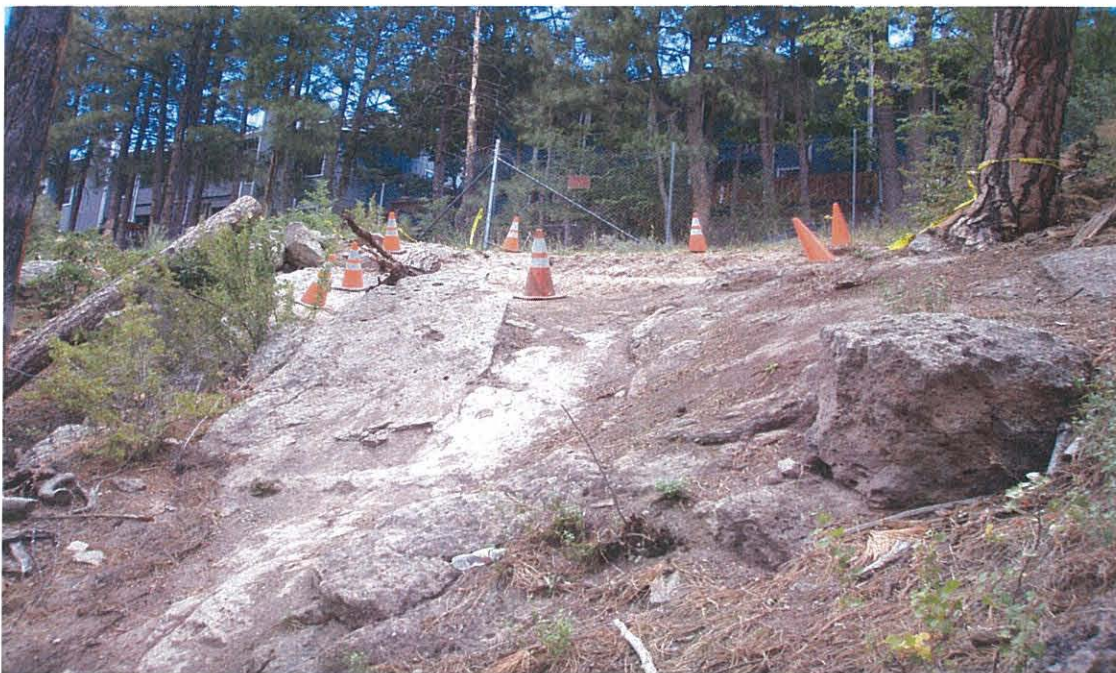
View of the excavation in the outfall area, looking northeast toward Timber Ridge Condominiums
