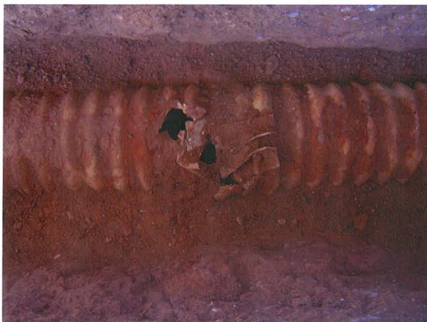
Photo 2. Break in old culvert.
