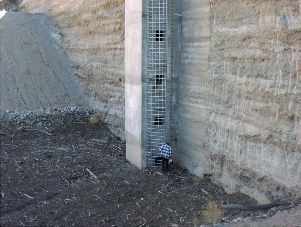
Figure 9. Inlet tower taken from north bank of reservoir to show spacing of openings.
